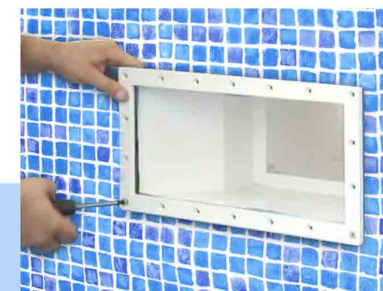
8. 泳池功能件安装 (水口、水下灯等) Installation of hydraulic accessories (water inlet/outlet, lights, etc.)
